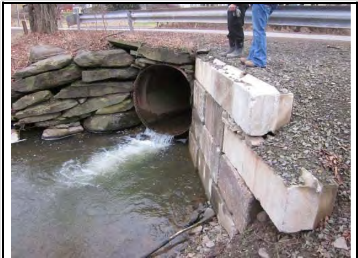
Photo 1: Looking upstream from left streambank at culvert outfall and failing head walls.
