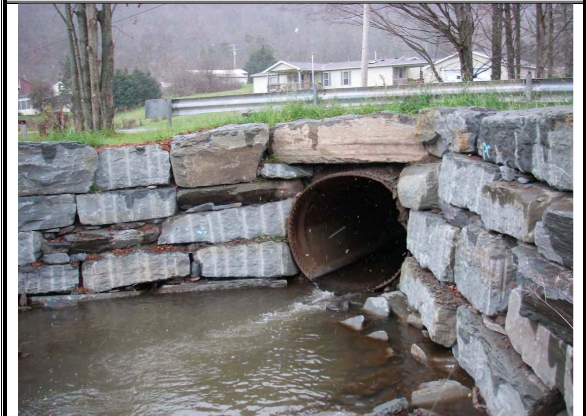
Photo 2: Looking upstream from left streambank after construction of stacked rock headwalls and plunge pool.
