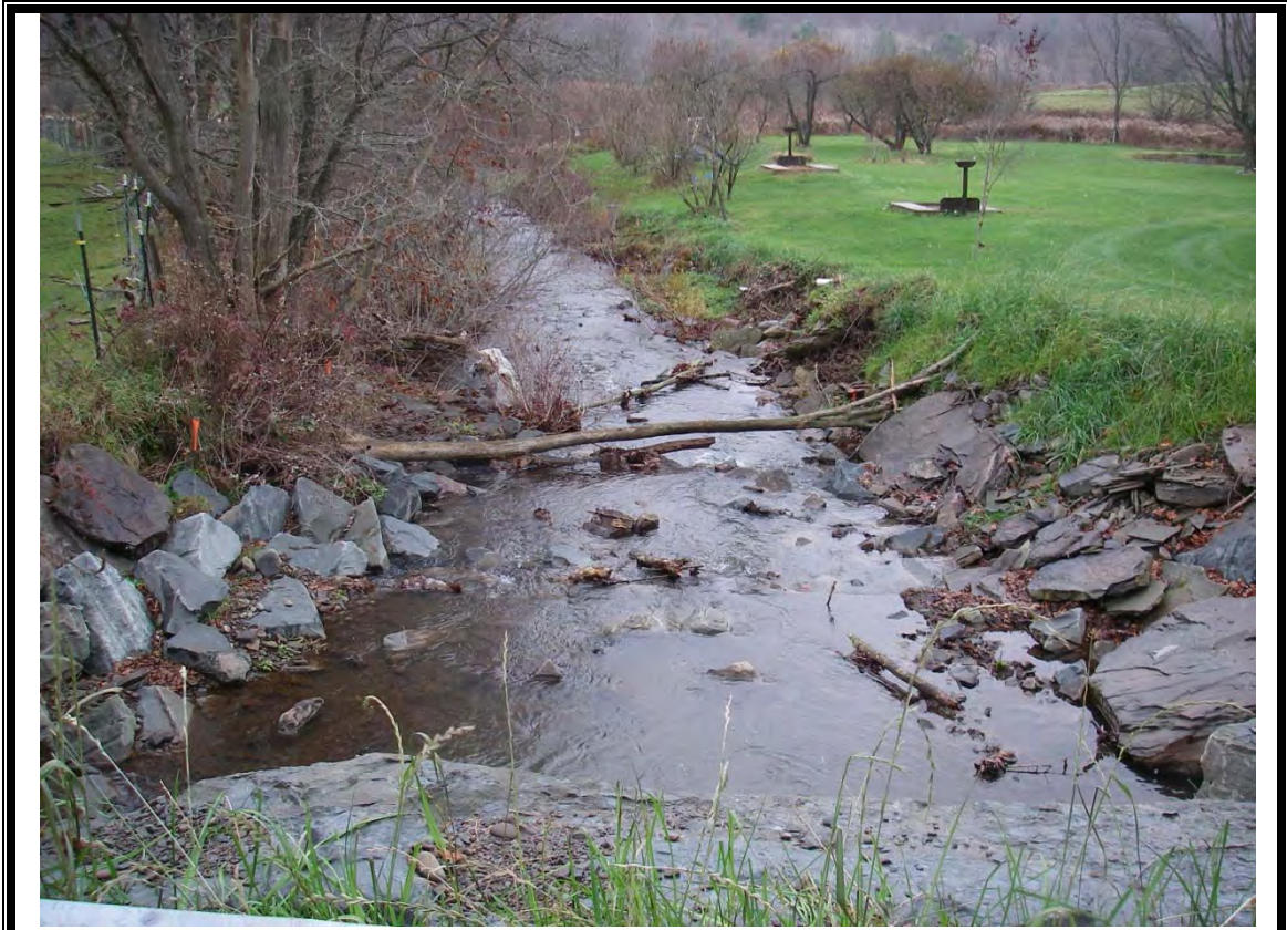
Photo 5: Looking downstream from Gosper Road after construction of plunge pool for culvert outlet protection.
