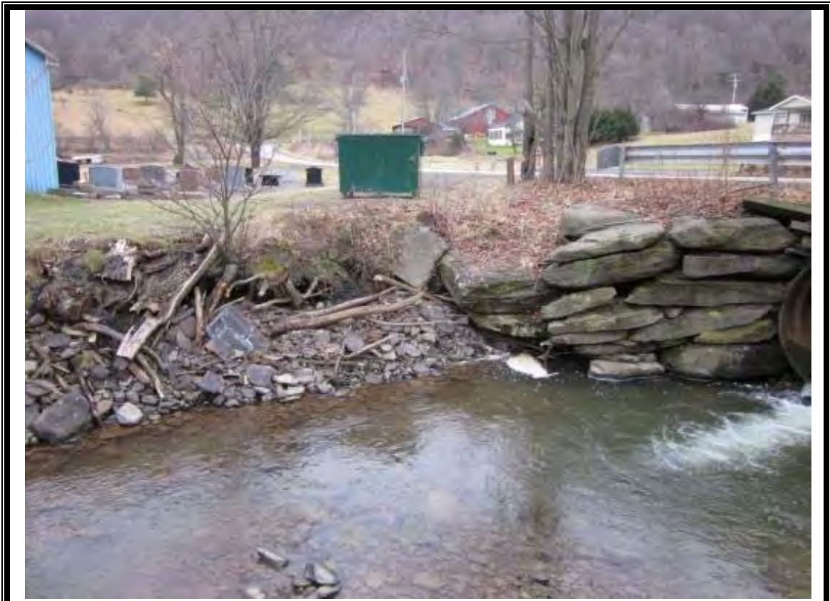
Photo 3: Looking upstream from left streambank at culvert outfall and failing head walls.
