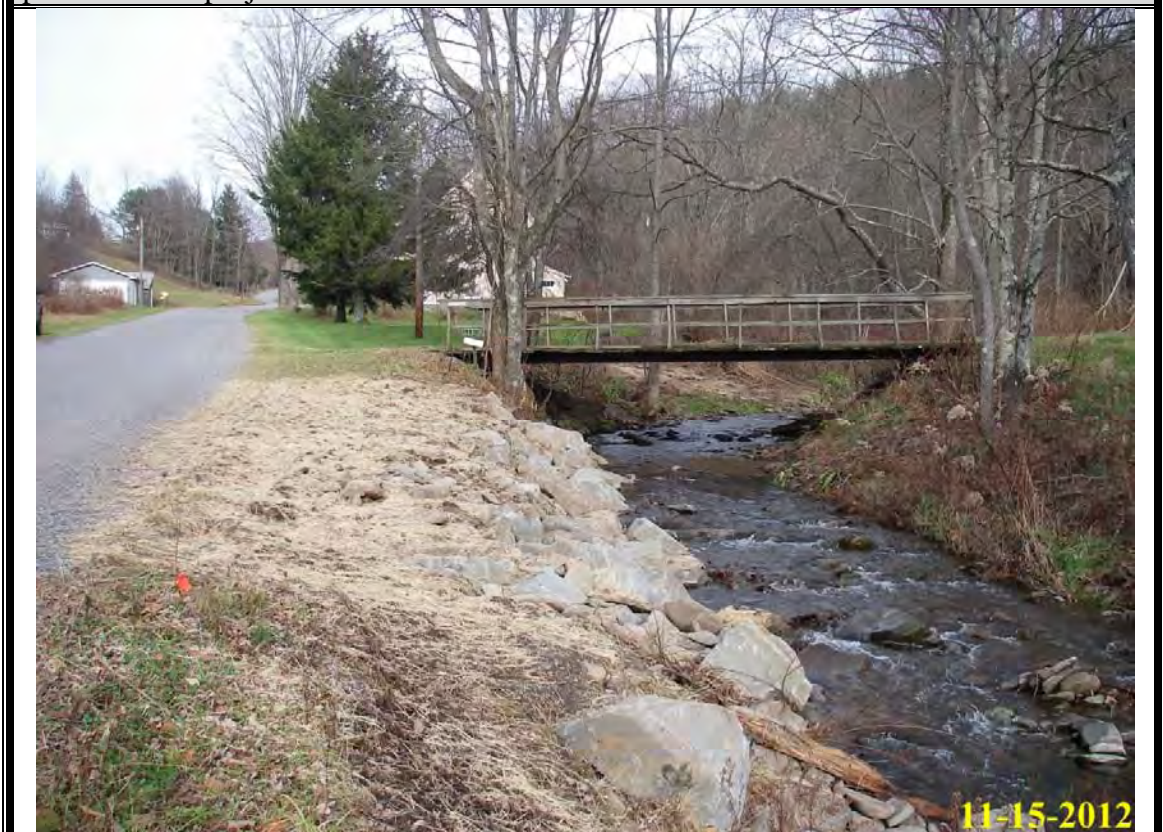
Photo 10: After construction, looking upstream from right streambank at lower portion of the project.
